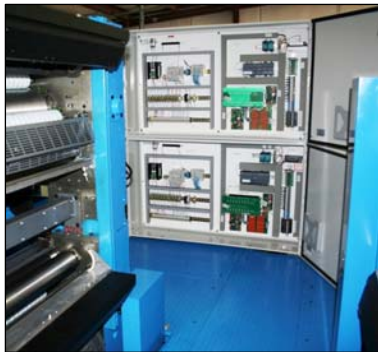
New Electrical Controls
